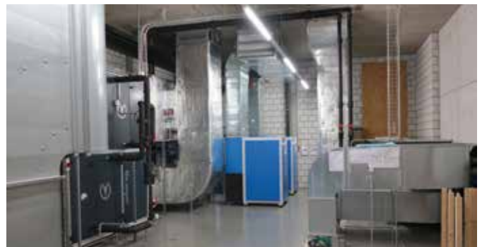
Two new compressors in the spacious ventilation room. Photo: Márton Varga, Topmotors
