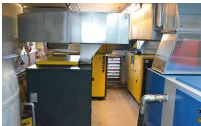
Four old compressors in the old utility room. Photo: Alain Chappatte, Energie du Jura
