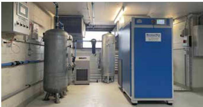
The same utility room, with only one new compressor. Photo: Michael Broccard, Schrad'air Compresseurs SA
