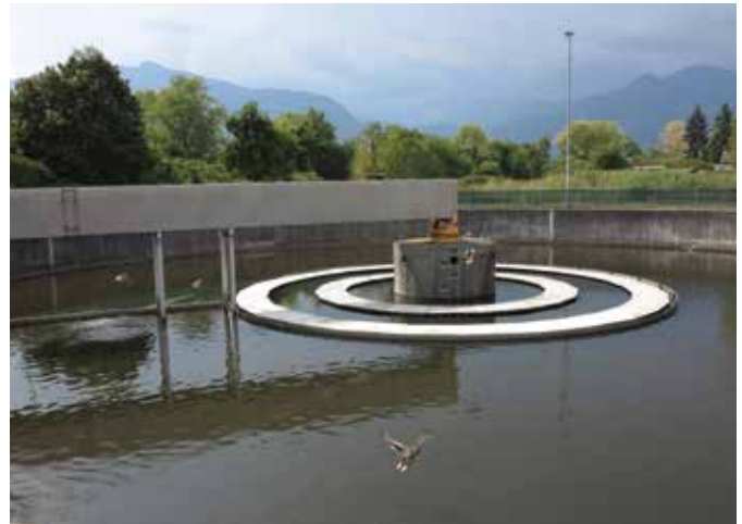
Clarification basin at ARA Foce Maggia. Photo: Topmotors
