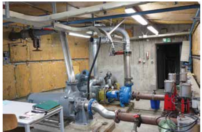
The pumping station with the two sludge pumps. Photo: Topmotors
