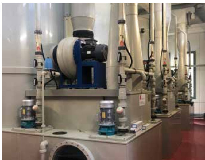
The waste air purification system. Photo: PAMP
