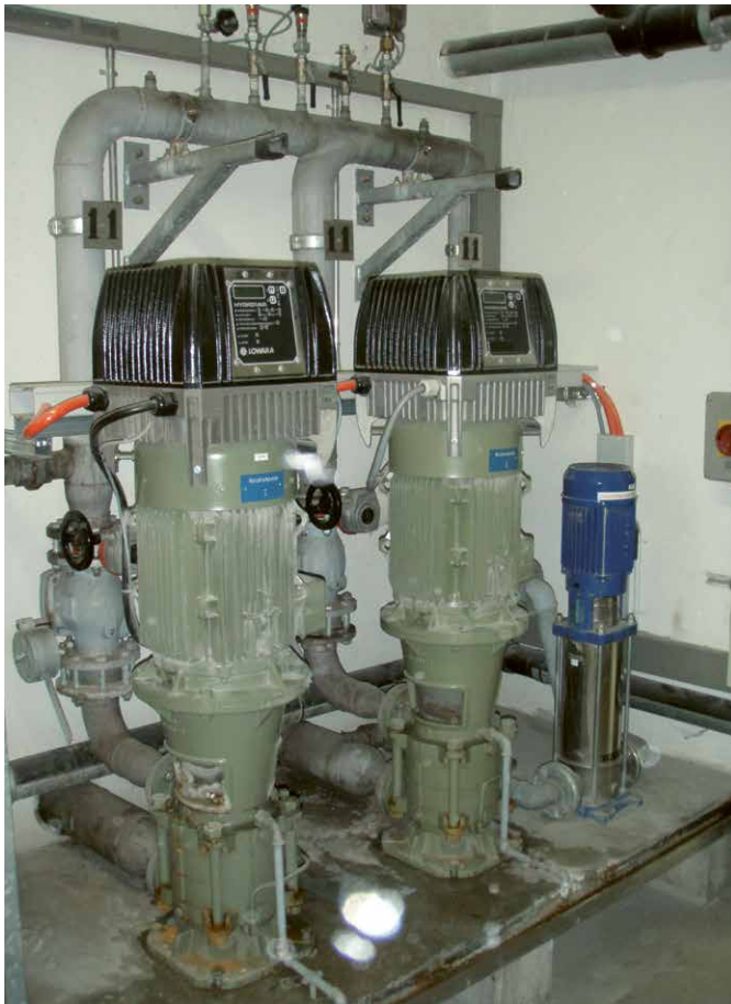
Former high-pressure installation with 2 Häny 4504/3 pumps (from 1992) and 1 Lowara SV808 pump for maintaining the pressure (2001).
