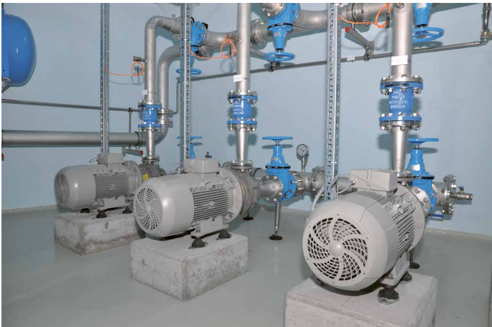
New system with redundant pumps and renewed pipework. Picture: Stefan Hartmann, Presseladen.
