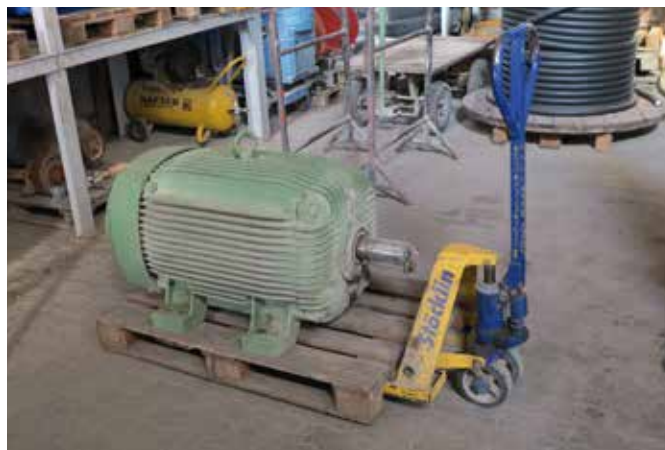
The old motor, kept as a back-up
