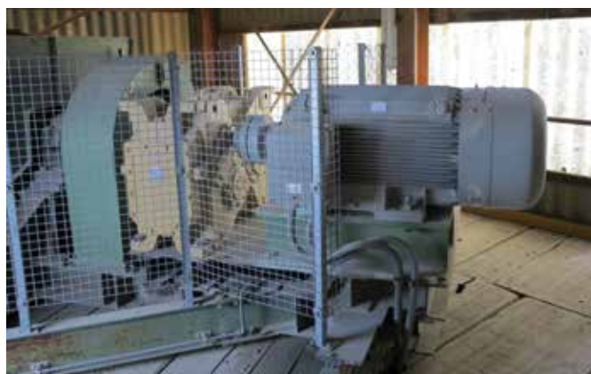
The new motor in operation
